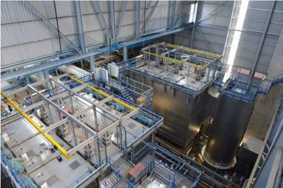
Plate 3.7: Typical Bag Filter House
