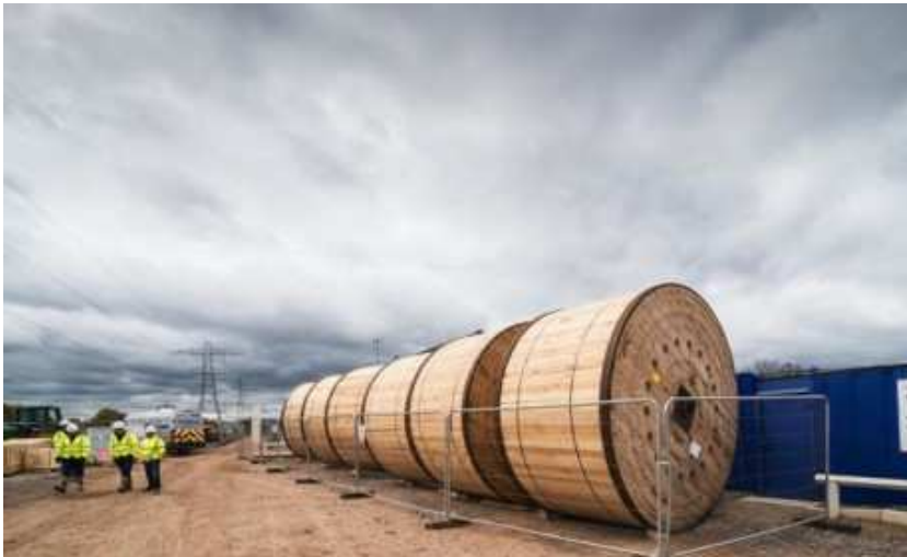
Plate 3.20: Example of 132kV Cable Drum Storage in Cable Route Temporary Construction Compound
