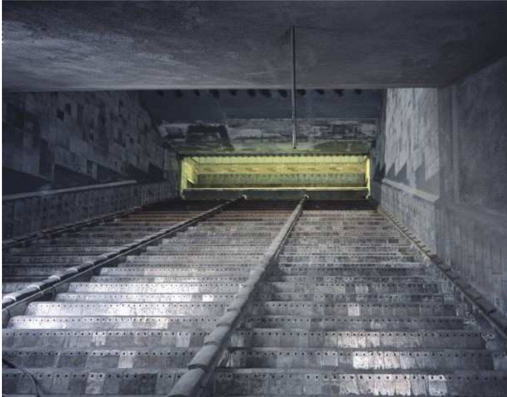
Plate 3.6: Typical Combustion Chamber and Grate
