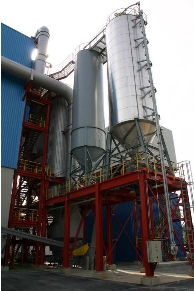
Plate 3.11: Typical Storage Silos
